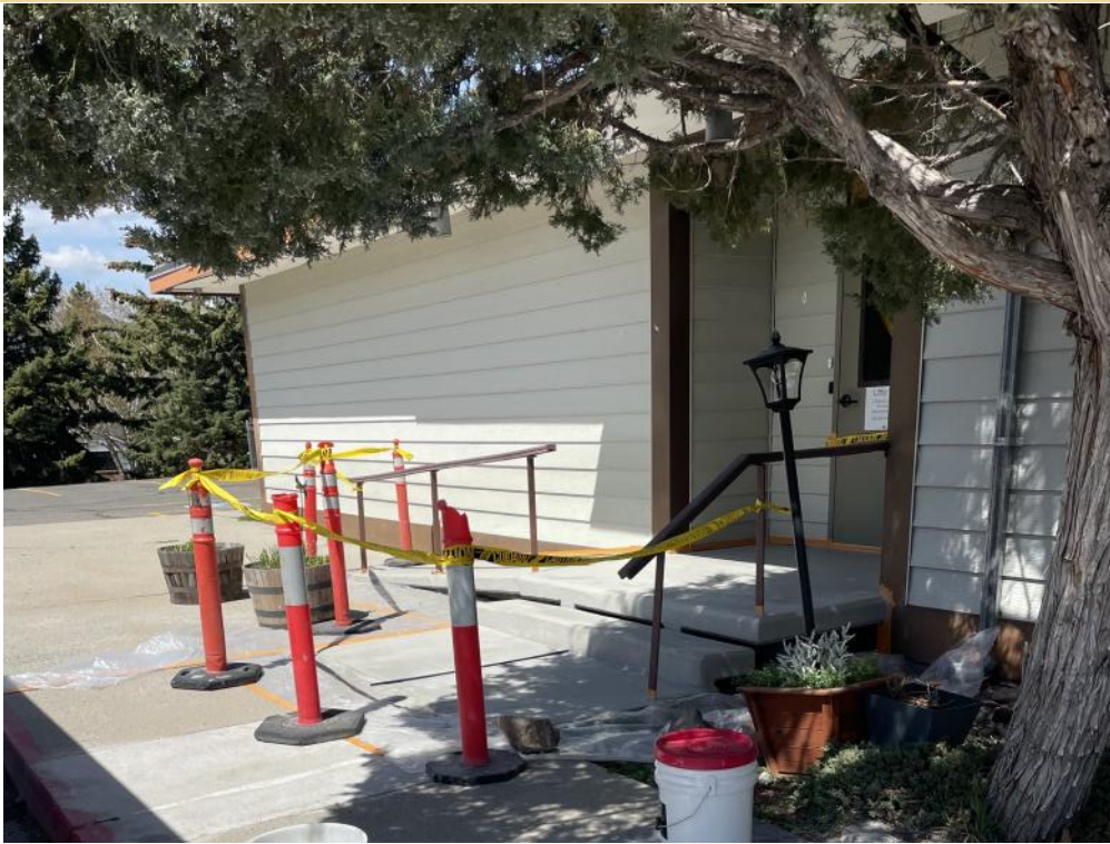
The stairs and ramp to the daycare got a much needed tune-up last week.
